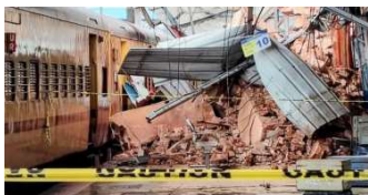
Heavy rain triggered the partial collapse of the 150-year-old heritage clock tower onto Platform No. 2 of the station. K. RAGESH
