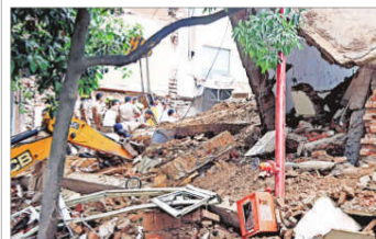
At the site of building collapse, Chandigarh, Saturday. KAMLESHWAR SINGH
